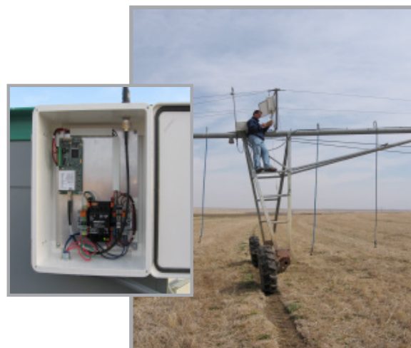
Figure 2 and 3 Installation of a control box with a wireless M2M communication device.
